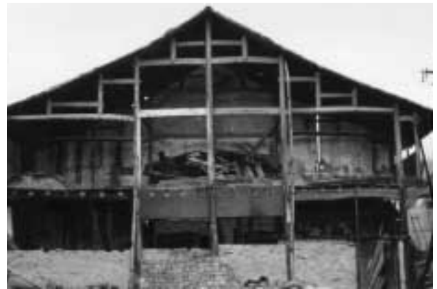
Figure 2.4. By tripling the depth of a dwelling and increasing the height of columns, a second floor is made possible. The wooden framework structure of this dwelling, clearly evident because the building is being dismantled, is discussed in Chapter 3. Lubucun, Shuidong xiang , Lishui xian , Zhejiang. [RGK photograph 1987.]
