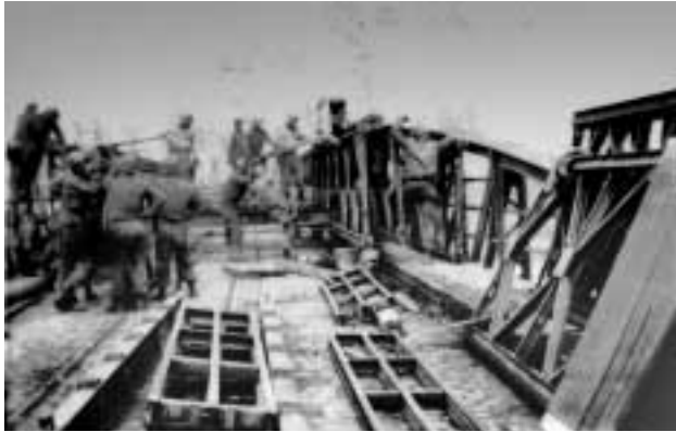
(Above) 348th Combat Engineering Battalion Company A working on bridge spanning the Sieg River outside Siegburn, March 1945.
